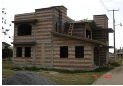
Figure 1. Most common configuration of combined and confined masonry: 3 courses of bricks alternate with 1 course of concrete blocks.
