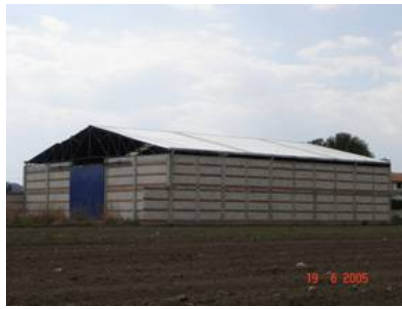
Figure 3. Combined and confined masonry warehouse: 3 courses of bricks alternate with 3 courses of concrete blocks.
