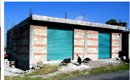
Figure 7. Combined and confined masonry store: 2 courses of bricks alternate with 2 courses of concrete blocks.
