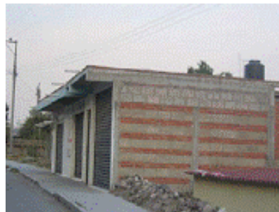
Figure 6. Combined and confined masonry store: 2 courses of bricks alternate with 1 course of concrete blocks.
