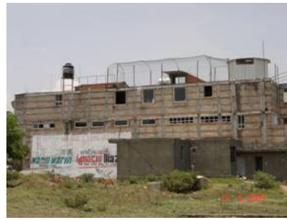
Figure 4. Three-story combined and confined masonry apartment building: 3 courses of bricks alternate with 2 courses of concrete blocks.
