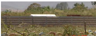
Figure 5. Combined and confined masonry fence: 2 courses of bricks alternate with 3 courses of concrete blocks.
