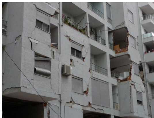
Figure 2. Earthquake-damaged infill walls, some of which have fallen out of the building.
