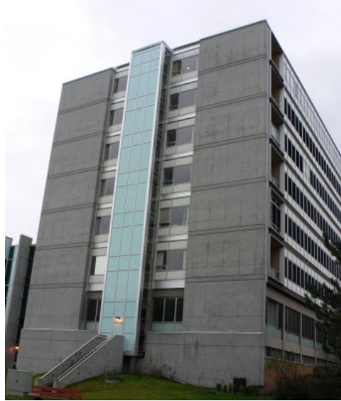
Figure 2. The seismic retrofit of this hospital building included two new structural walls and foundation at each end.
