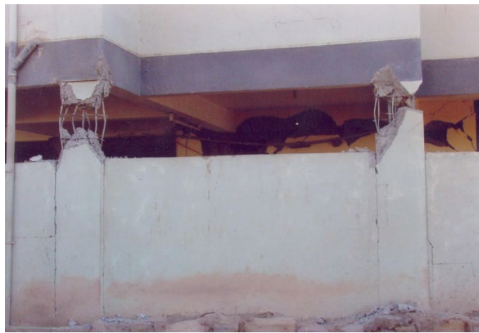
Figure 4. Earthquake-damaged short columns.
