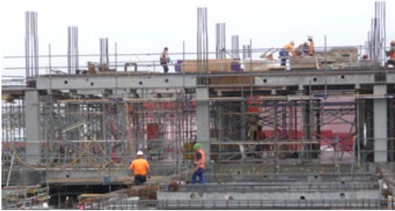
Figure 3. An engineer needs to regularly visit construction sites like this to ensure construction is in accordance with the plans and specifications.
