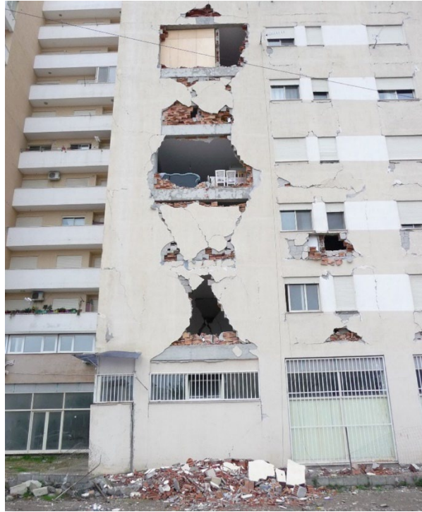
Figure 2. An example of an earthquake damaged building where the infill walls have not been carefully designed to allow for forces and movements during an earthquake.
