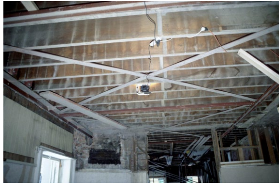
Figure 5. A timber floor of a masonry building is strengthened for earthquake resistance by steel bracing underneath it.
