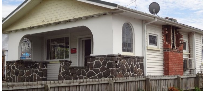
Figure 3. A brick chimney has broken off at roof level and fallen. Most of the remaining chimney is damaged (N. Allaf).
