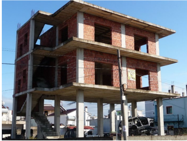
Figure 5. A typical soft story building where the ground floor is the weakest.
