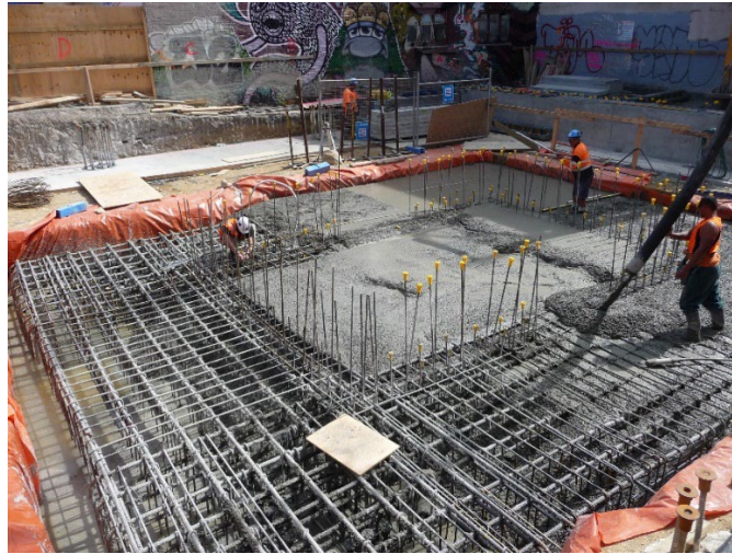
Figure 3. The foundations of a building under construction. Engineers have followed codes to determine the amount of reinforcing steel and its correct location.
