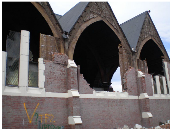
Figure 4. An earthquake has destroyed most of the brick cladding and glazing of this building.
