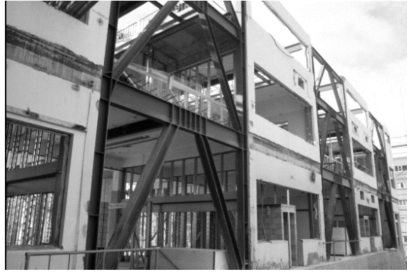
Figure 4. Bays of steel bracing are inserted into this building as part of the retrofit.
