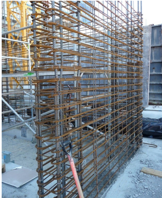
Figure 1. Severe damage during an earthquake could occur if several reinforcing bars are missing from this reinforced concrete wall.
