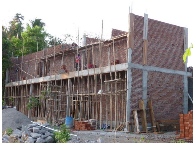
Figure 3. Conventional heavy construction using reinforced concrete and masonry - in this case, confined masonry construction.
