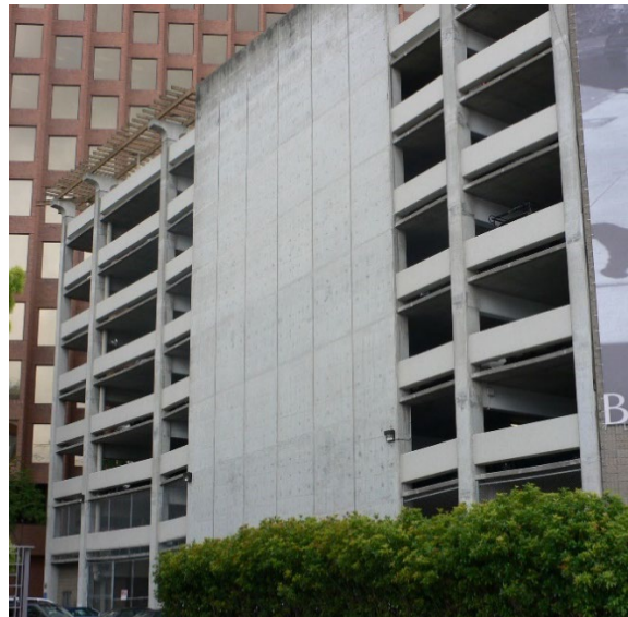
Figure 4. A reinforced concrete structural wall resists forces acting along the length of the building. There should be another wall on the other side of the building.
