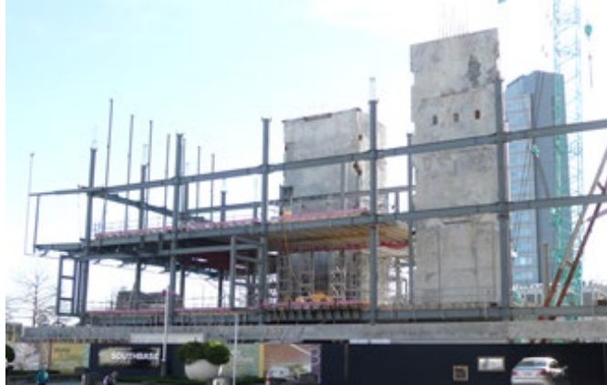
Figure 3. A building under construction. Most of the earthquake forces in both directions are resisted by reinforced concrete structural walls. In this case, some assistance is also provided by a perimeter steel moment frame.
