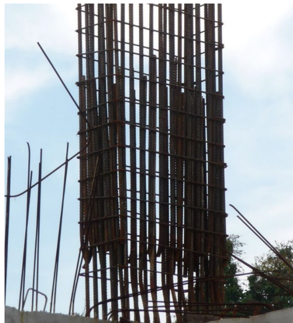
Figure 2. The reinforcement of this column does not comply in numerous ways with the local codes and standards. During a moderate to large earthquake, it will be seriously damaged.
