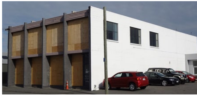
Figure 1. An earthquake damaged building. The strength and stiffness of the long white-colored masonry walls have prevented damaged. A more flexible structural system acting across the building has led to larger movement and damage to the front façade. It is temporarily covered with sheets of plywood.
