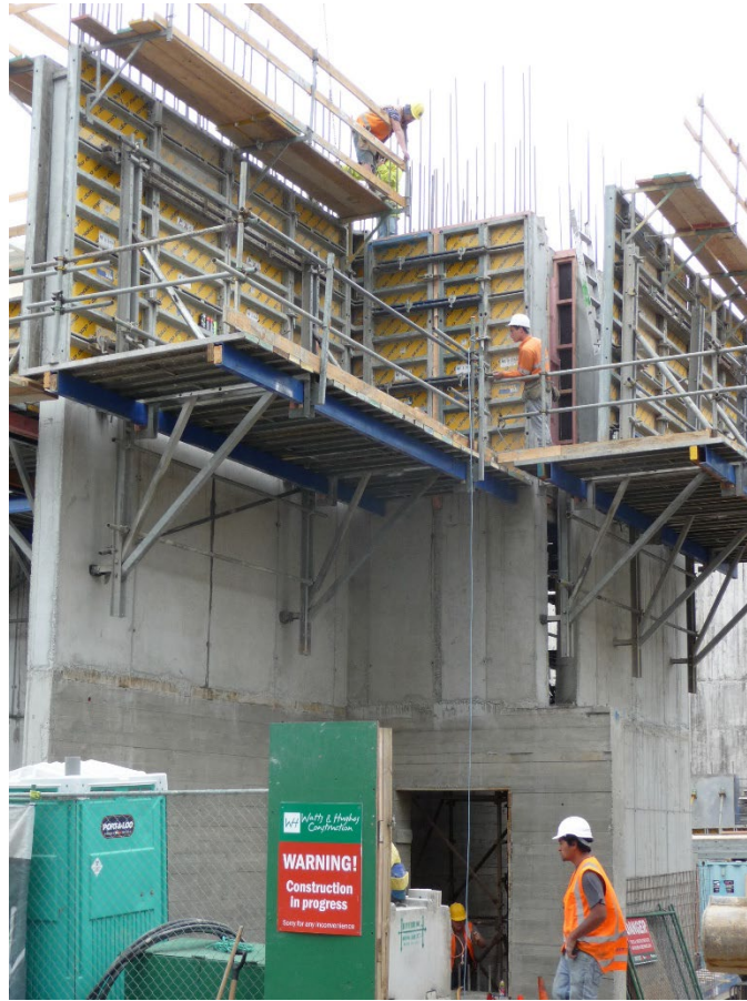
Figure 2. During both design and construction these reinforced concrete walls were checked by engineers to ensure the structural design was sound and that construction was in accordance with the plans.
