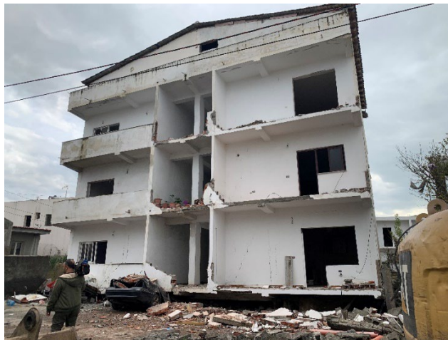
Figure 4. This soft story building lost its ground floor during a moderate earthquake (N. Vesho).
