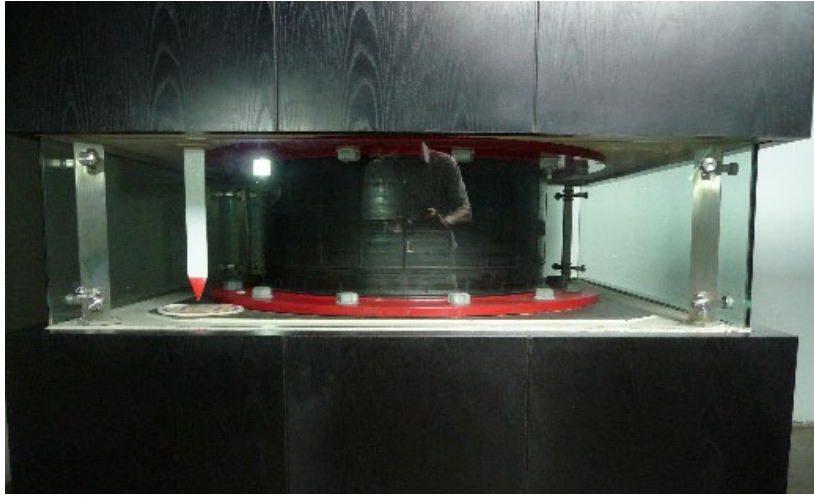
Figure 4. A circular rubber bearing containing many thin steel plates is located between the bottom of every column and its foundation to isolate the building from horizontal earthquake shaking.
