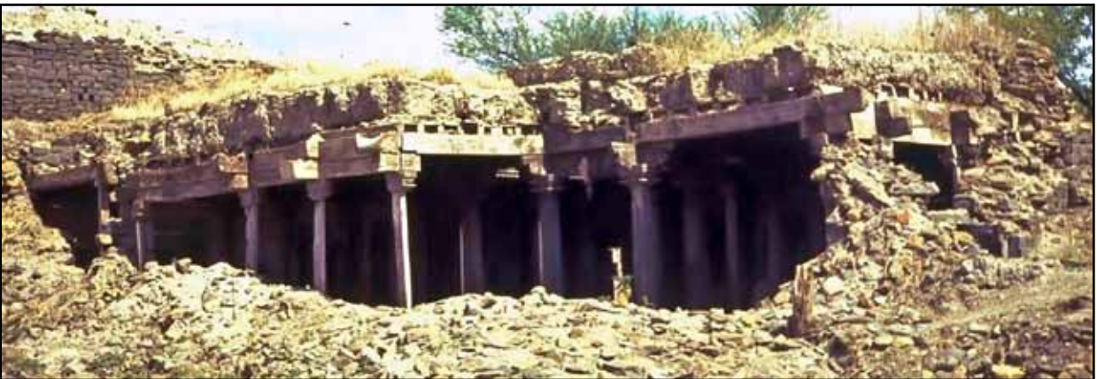
Figure 2.19 Wall collapse in the 1993 Maharashtra, India, earthquake. Stone masonry buildings had timber roofs with heavy mud overlays (photo: S. Brzev)
