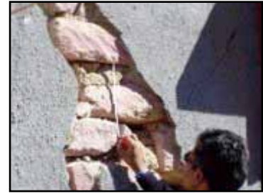
Figure 2.36 A stone masonry wall with thick mud mortar (thickness on the order of 80 mm) in the area affected by the 2001 Bhuj, India, earthquake (photo: J. Arlekar)
