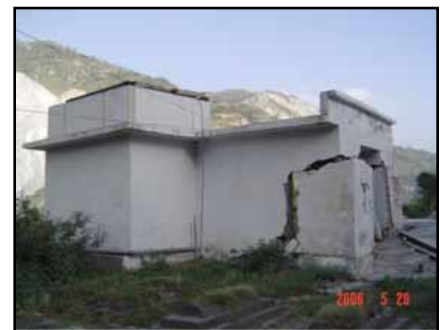
Figure 2.38 Soil spreading in the 2005 Kashmir, Pakistan, earthquake - note wide cracks in the walls (source: Bothara and Hiçyılmaz 2008)
