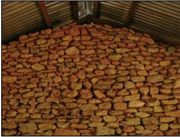
Figure 2.31 A tall gable wall in Nepal that is at risk due to the absence of a roof connection (photo: Smart Shelter Foundation)
