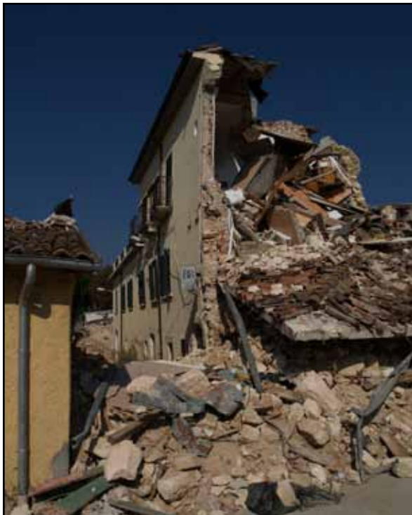
Figure 2.1 Extensive damage to stone masonry buildings in the 2009 L'Aquila, Italy, earthquake (photo: T. Schacher)
