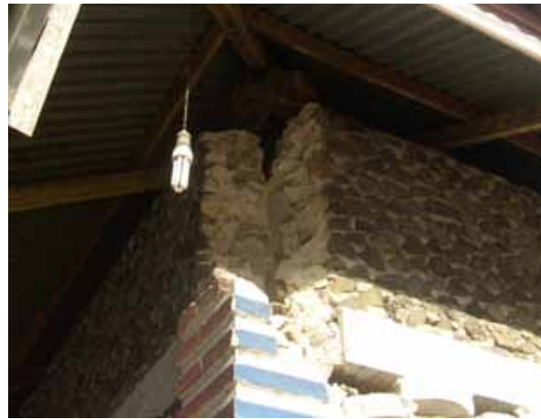
Figure 2.9 Damage at a wall intersection of a single-story stone masonry building in the 2009 Padang, Indonesia, earthquake (note absence of bands at lintel and roof levels) (source: Bothara et al. 2010)
