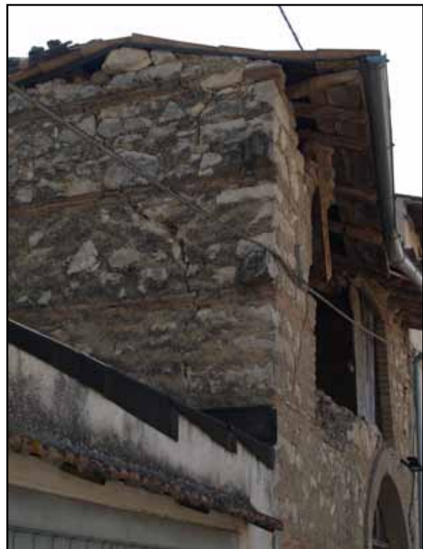
Figure 1.30 A stone masonry wall with brick bands in L'Aquila, Italy (photo: T. Schacher)
