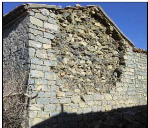
Figure 2.22 Delamination of a stone masonry wall in the 2000 Beni-Ouartilane, Algeria, earthquake (photo: M. Farsi)
