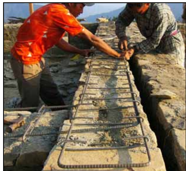
Figure 3.18 Properly bent steel links for RC band construction (photo: Smart Shelter Foundation)
