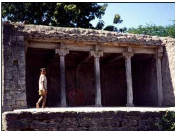
Figure 1.12 A timber roof structure with mud overlay in Maharashtra, India (photo: S. Brzev)
