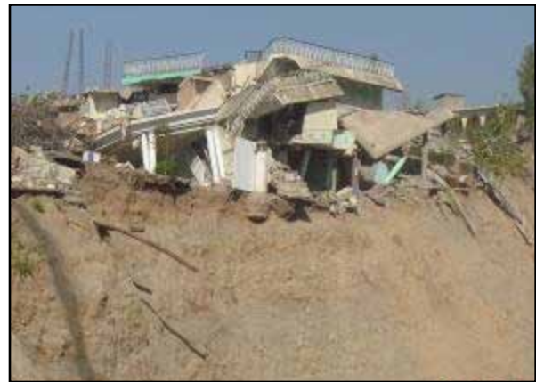
Figure 3.3 A building damaged by a landslide in the 2005 Kashmir, Pakistan, earthquake (source: Bothara and Hıçyılmaz 2008)
