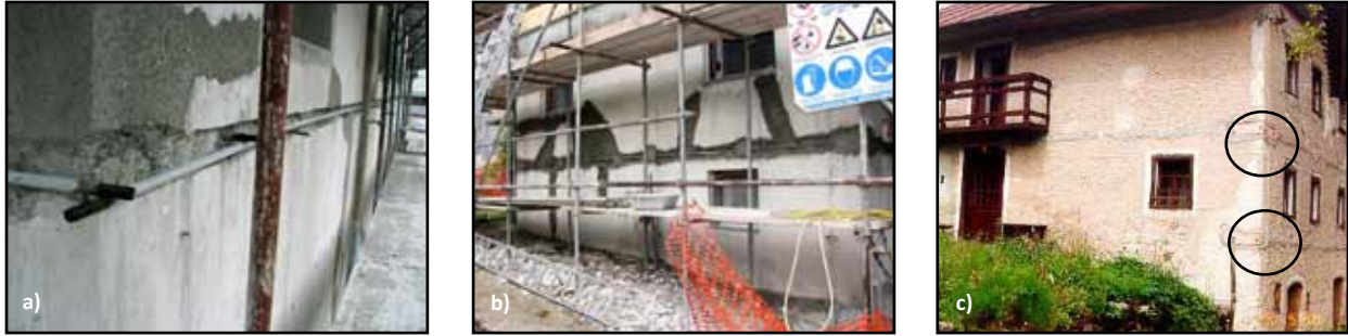
Figure 4.4 A field application of ties in Slovenia: a) and b) installation of steel ties after the 1998 Bovec, Slovenia, earthquake (note that anchorage end-plates are yet to be attached), and c) an example of a retrofitted building (photos: M. Lutman)
