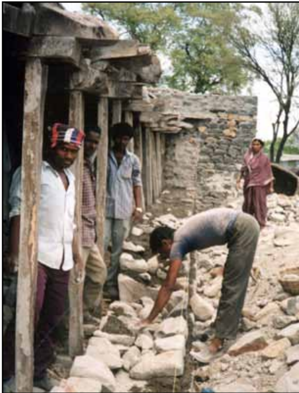
Figure 1.23 Construction of an uncoursed random rubble stone wall in Maharashtra, India (photo: S. Brzev)
