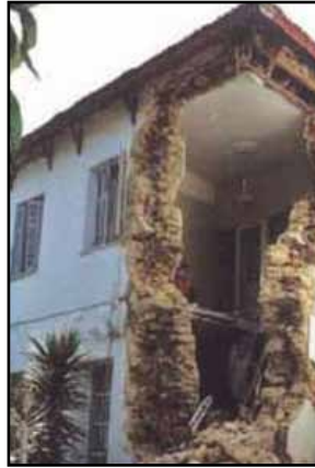
Figure 2.8 Disintegration of stone masonry walls in Greece (source: WHE Report 16)
