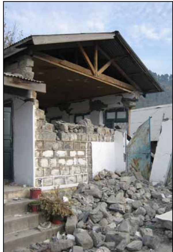
Figure 1.13 Timber truss roof structure in the area affected by the 2005 Kashmir earthquake in Pakistan (source: M. Tomazevic 1999)
