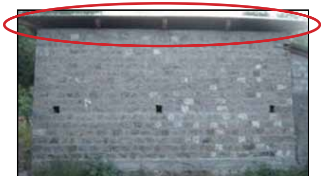
Figure 2.10 A stone masonry building in Muzzaffarabad was undamaged in the 2005 Kashmir, Pakistan, earthquake; this was attributed to the presence of an RC band at the eaves level (photo: J. Bothara)
