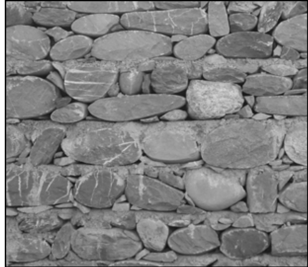
Figure 1.27 Stone masonry wall built using round river stone boulders with shaped exterior surfaces near Balakot, Pakistan (photo: T. Schacher)
