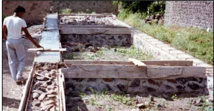
Figure 3.39 Construction of an RC plinth band using large stone rubble (also known as "stone-crete") (photo: S. Brzev)
