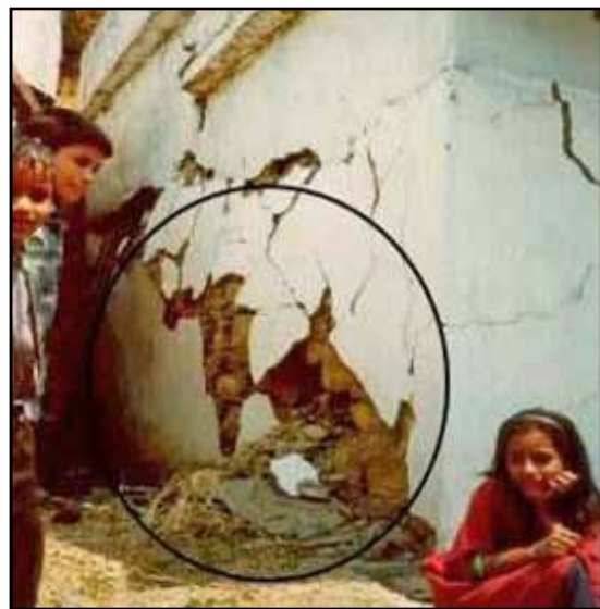
Figure 2.35a Localized wall failure caused by irregular stones (source: WHE Report 74)
