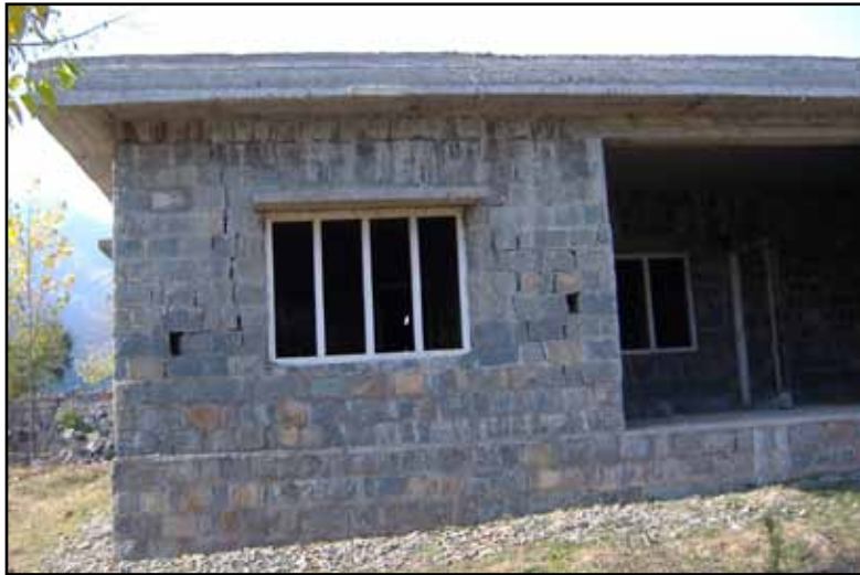
Figure 1.14 A stone masonry building with an RC slab roof in Pakistan (photo: J. Bothara)
