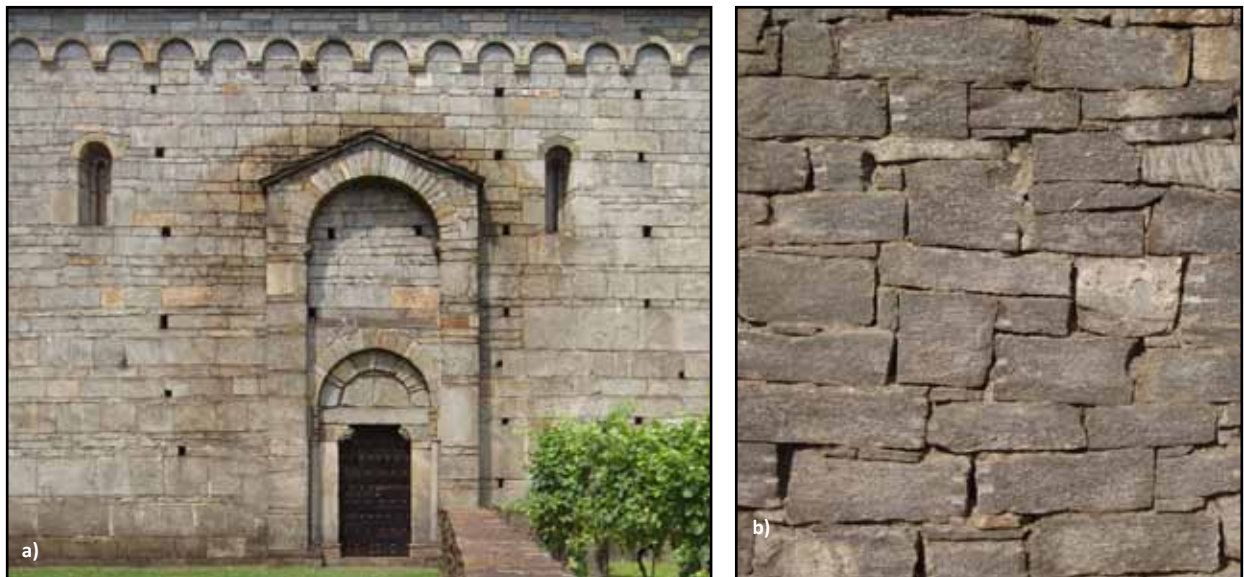
Figure 1.32 Dressed stone masonry construction in Southern Switzerland: a) a typical building in Giornico, and b) a detail of the exterior (photos: T. Schacher)
