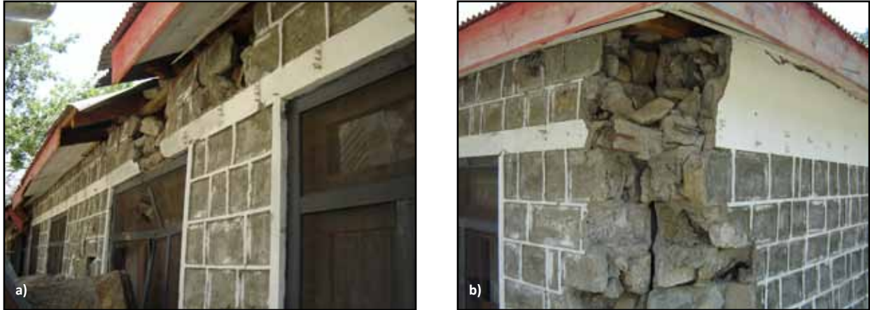
Figure 2.11 A stone masonry building with an RC lintel band that survived the 2005 Kashmir earthquake in Pakistan: a) the building suffered only moderate damage in the top portion, and b) separation at the wall intersection took place in spite of the band (note inadequate anchorage of the band reinforcement) (photos: Builders Without Borders)
