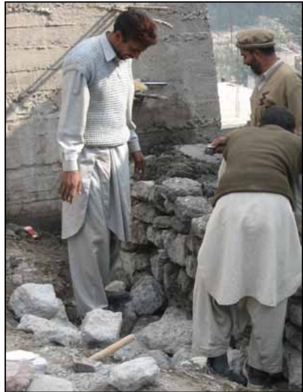
Figure 1.24 Construction of an uncoursed random rubble stone wall in Pakistan after the 2005 Kashmir earthquake (photo: M. Tomazevic)
