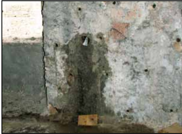
Figure 4.27 Grouting an existing stone masonry wall in Slovenia - note uniformly distributed holes at the location where grout is to be injected (photo: M. Lutman)
