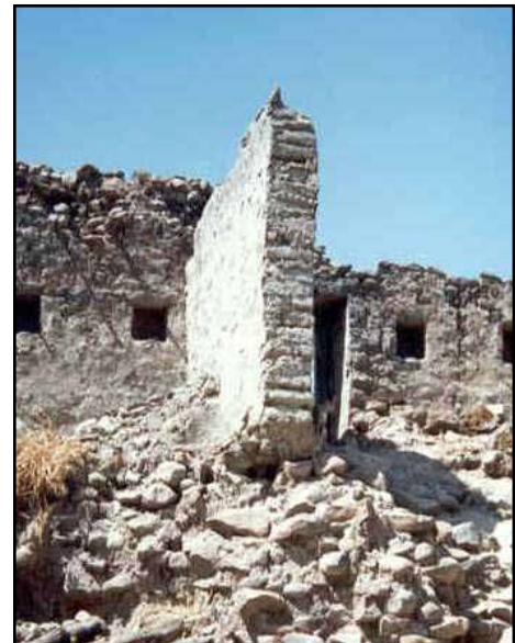
Figure 1.18 A wall without foundations in the area affected by the 1993 Maharashtra, India, earthquake (photo: S. Brzev)
