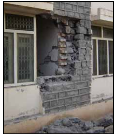
Figure 2.37 Vertical cracking at a wall intersection due to the 2005 Kashmir, Pakistan, earthquake due to absence of connection between the intersecting walls, a stone masonry and a brick-masonry wall (source: Bothara and Hiçyılmaz 2008)
