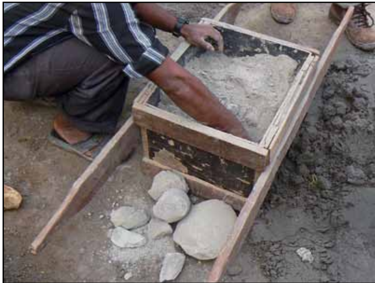
Figure 3.43 Cement with large lumps should not be used for construction (photo: Smart Shelter Foundation)
