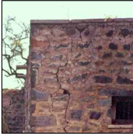
Figure 2.7 Vertical crack in a stone masonry wall due to the 1993 Maharashtra, India, earthquake (photo: S. Brzev)
