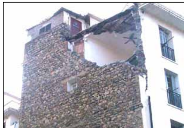
Figure 2.25 Out-of-plane collapse at the top floor of a stone masonry building in the 2003 Boumerdes earthquake in Algeria (photo: M. Farsi)
