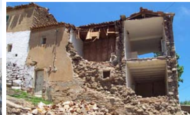
Figure 5F: Totally collapsed stone masonry building in Dellys (Boumerdes) in the May 21, 2003 earthquake
