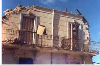
Figure 5B: Typical Earthquake Damage: Collapsed Roof of a Masonry Building (1989 Tipaza Earthquake)
