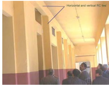
Figure 6B: Seismic Strengthening Techniques: An Example of a Strengthened Building with Vertical and Horizontal RC Ties at the First Floor Level
