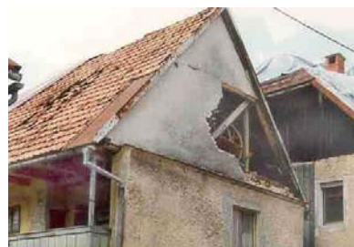
Figure 6B: Out-of-plane gable collapse
