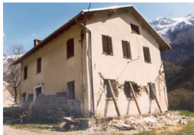
Figure 6A: a Photograph Illustrating Typical Earthquake Damage in the 1998 Bovec earthquake
