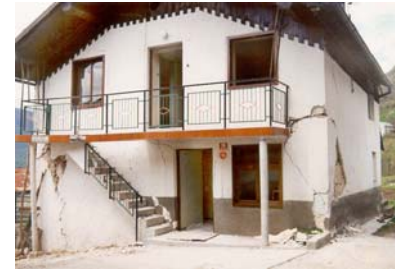
Figure 5A: an Illustration of Key Seismic Deficiencies - lack of structural integrity results in wall dislocation and corner damage
