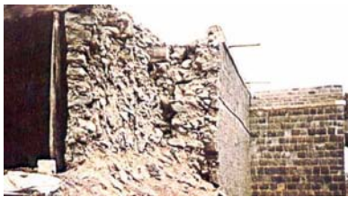
Figure 6C: Typical Earthquake Damage - Delamination of the Exterior Wall Wythe (the interior wythe remained undamaged due to restraint provided by timber posts), 1993 Killari Earthquake
