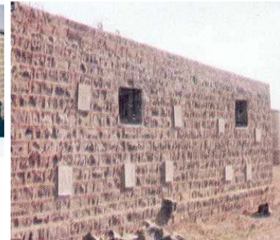
Figure 7H: Seismic Strengthening - An Example of a Retrofitted Building (note through-stones and RC lintel band)
