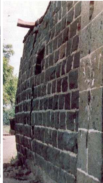
Figure 6B: Typical Earthquake Damage - Partial Collapse of the Exterior Wall in the 1993 Killari earthquake (Salegaon Village, Source: GSI 1996)
