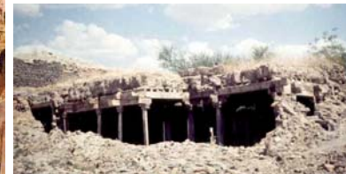
Figure 5E: Seismic Deficiency - Excessive Mud Overlay Atop the Roof
