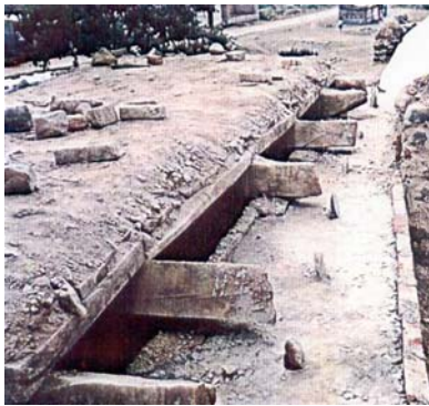
Figure 7C: Seismic Strengthening - Installation of a Bandage at the Lintel Level (an alternative to the installation of RC band) Source: GOM 1998
