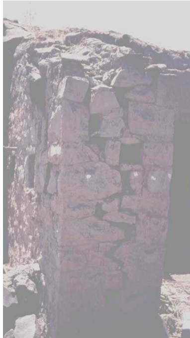
Figure 6A: Massive Collapse of Stone Masonry Buildings in the 1993 Killari Earthquake (Yelvat Village, Source: GSI 1996)
