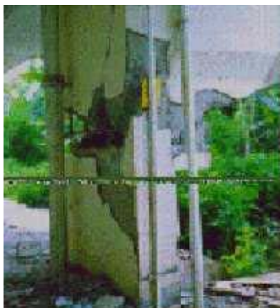
Figure 5A: A Photograph Illustrating Typical Earthquake Damage in the Labuan, Sabah (M5.8) of 26 May 1991
