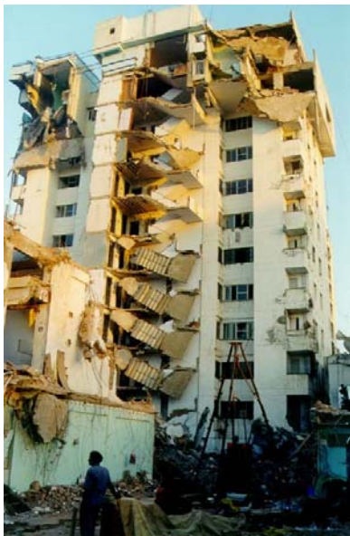
Figure 6A: A Photograph Illustrating Typical Earthquake Damage
