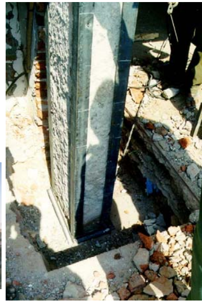
Figure 6F: Failure of Column Below the Beam-Column Joint Due to Short Column Effect
