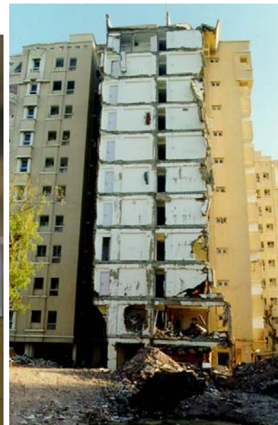
Figure 6C: Severe Damage and Plastic Hinging of Ground-Floor Column Due to Improper Confinement of Concrete and Lapping of Large Number of Longitudinal Bars
