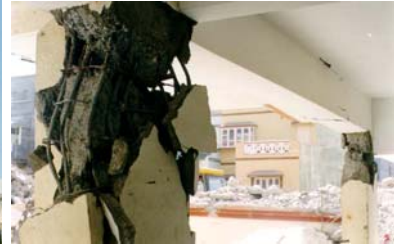
Figure 7C: Seismic Strengthening of Columns by Jacketing from Floor Level - Improper Technique (2001 Bhuj Earthquake)
