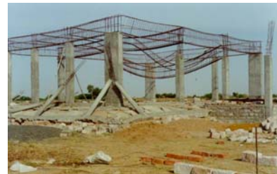
Figure 6L: Pancake Collapse of a Multistory Building Due to Weak Column-Strong Beam Design (2001 Bhuj Earthquake)
