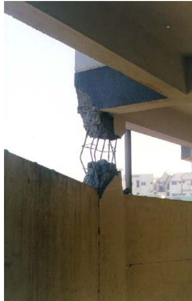
Figure 6B: Improper Reinforcement Detailing of Beam-Column Joint
