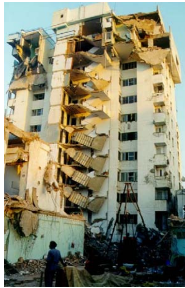
Figure 6H: Failure of Lower Two Stories of the Right Wing of an Apartment Building With Soft Story. Note that the Left Wing Without Soft Story is Apparently Undamaged (2001 Bhuj Earthquake)
