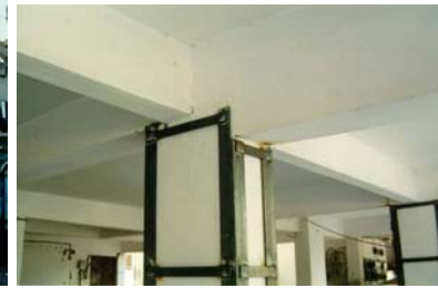
Figure 6I: Underutilization of Shear Capacity of Elevator Core Due to Improper Diaphragm Action of Slabs Resulted in Failure of an Apartment Building (2001 Bhuj Earthquake)
