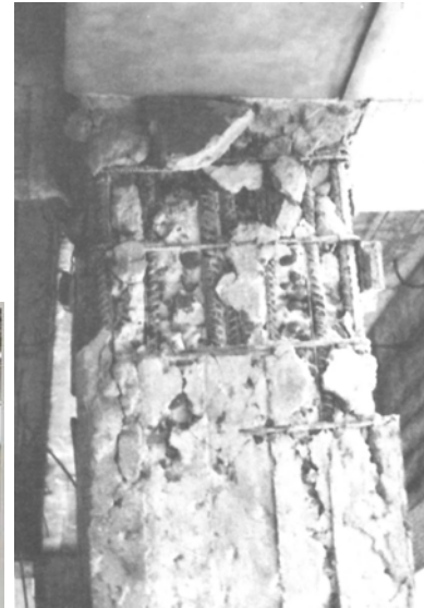
Figure 6C: San Antonio Hospital, close-up damaged in the 1985 Llole earthquake
