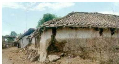
Figure 6C: Typical Earthquake Damage - Cracking and Separation of Walls in the 1997 Jabalpur Earthquake (Source: Sudhir K. Jain, IIT Kanpur)
