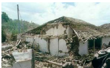
Figure 6B: Typical Earthquake Damage - Collapse of roof in the 1997 Jabalpur Earthquake (Source: Sudhir K. Jain, IIT Kanpur)
