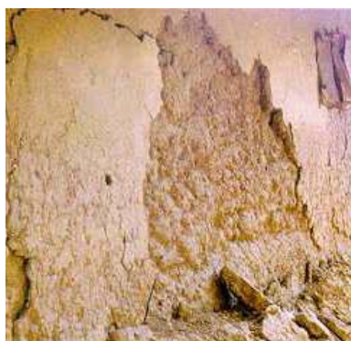
Figure 6: Typical Earthquake Damage
