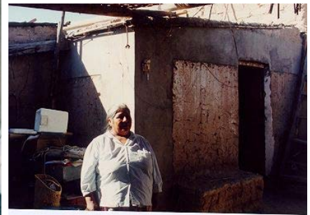
Fig. 18: Adobe house reinforced with strips of wire mesh, undamaged after 2001 earthquake in Moquegua.
