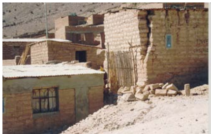
Fig. 16: Inspection after 2001 Earthquake in Moquegua: reinforced house without damage and neighboring unreinforced house with severe damage,
