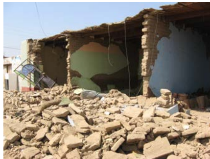
Fig. 20: Collapsed houses in the same block as the reinforced house of Fig. 19, after the 2007 earthquake in Ica.
