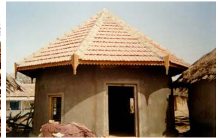
Figure 6B: A Photograph Illustrating Typical Damage (2001 Bhuj earthquake)
