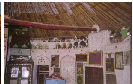
Figure 5A: A Photograph Illustrating Typical Earthquake Damage (2001 Bhuj Earthquake)
