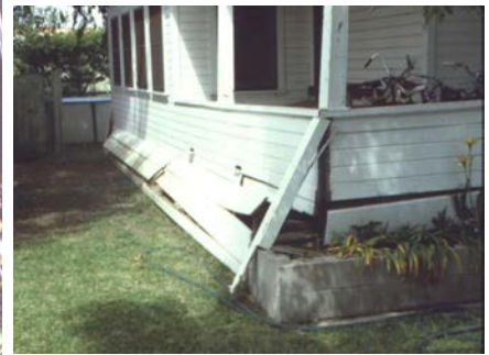
Figure 5C: The porch in front of this house has collapsed due to inadequate bracing, Whittier earthquake (Los Angeles), California, 1987
