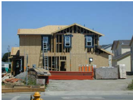
Figure 5A: Cripple wall failure, large house, Morgan Hill earthquake, California, 1994
