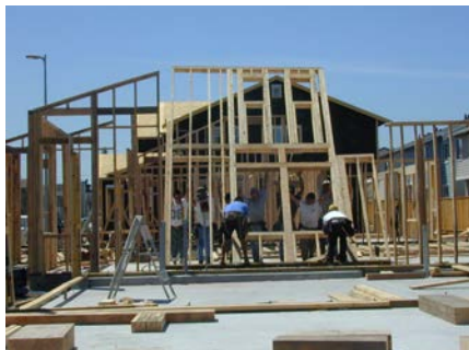
Figure 4D: House is framed, sheathed with particle board and windows are installed
