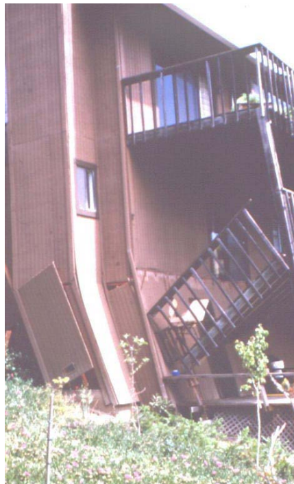
Figure 5B: Cripple wall failure detail, older house, Coalinga earthquake, California, 1983
