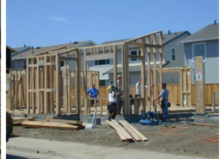
Figure 4C: Carpenters installing a stud wall which has been constructed on the concrete slab
