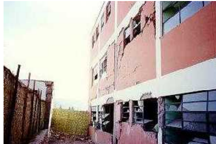
Figure 6: A Photograph Illustrating Typical Earthquake Damage
